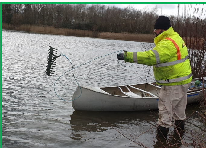
Waterweed removal trial; contractors using a water rake at the lake, March 2023
